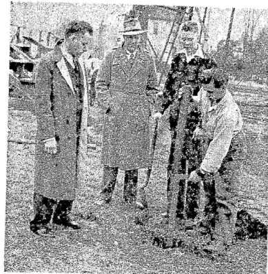
Ashton will have night ball games this summer and the repair work of the local bleachers is being carried out by the Agricultural class of the high school as a F. F. A. community service project. Shown above supervising the work (left to right) are: Glen Shippy, Ag. instructor, Paul E. Vaupel, principal, while students Don Kaecker and Verlis Voegler, are digging a post hole.
